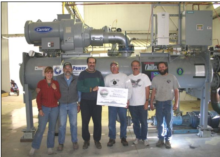
The Chena Chiller and project staff
