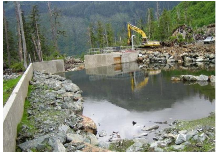
Prince of Wales Island, South Fork run-of-the-river hydroelectric project
