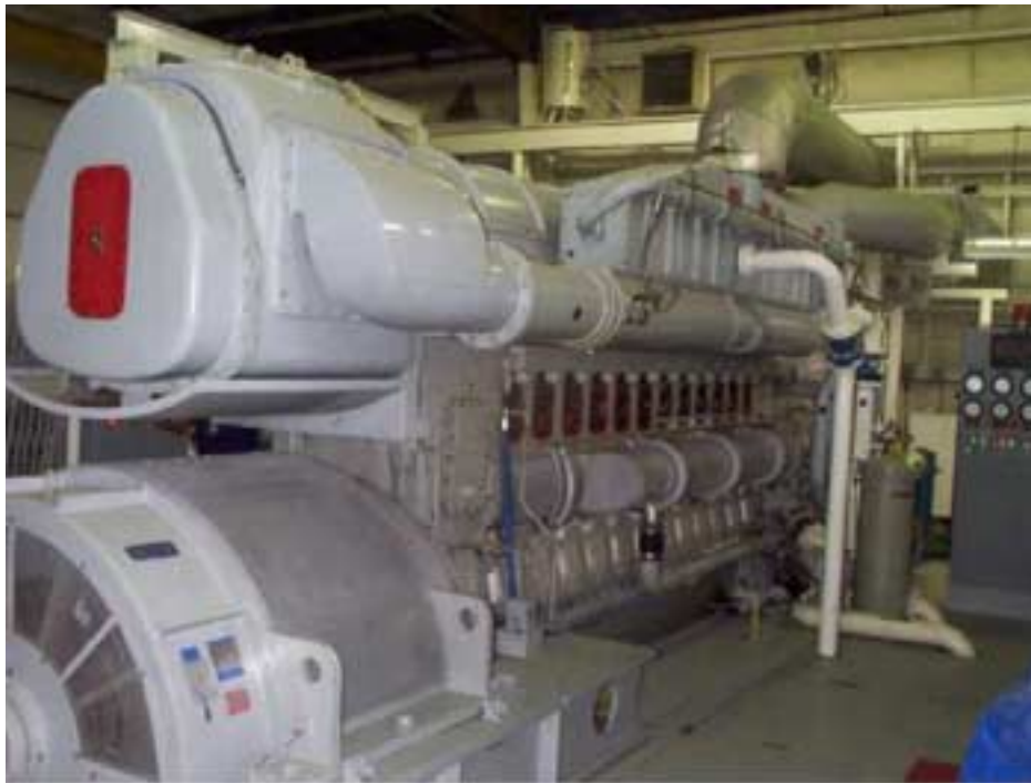
Figure 03 – UniSea Powerhouse, Fairbanks Morse No. 6 Engine-Generator
