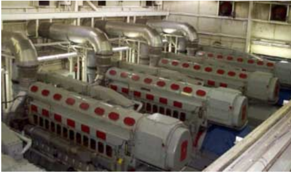
Figure 02 - UniSea Powerhouse, Fairbanks Morse Engine-Generators Nos. 4 through 1 (l-r)
